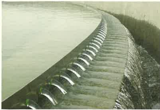
Water Supply & Waste Water
